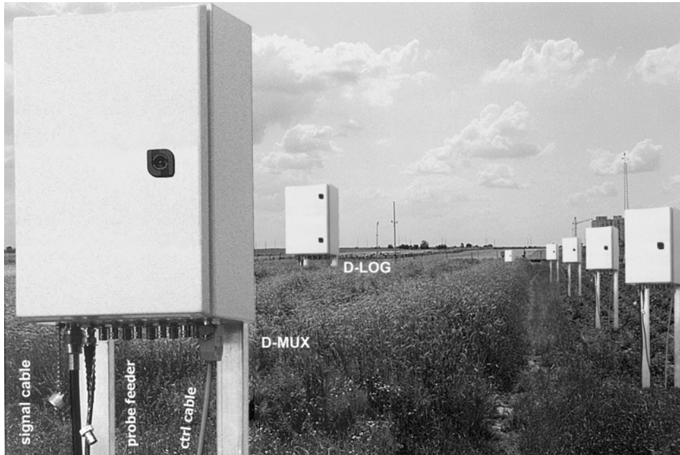
Fig. 12. An example of the D-LOG/10/mts-controlled stand incorporating six D-MUX/10/mts 2-nd level multiplexers. Maximum amount of the controlled FP/mts (or FP/m) probes is 60. For clarity only a single D-MUX was linked with the D-LOG and a single probe was connected to each D-MUX when taking the picture.
